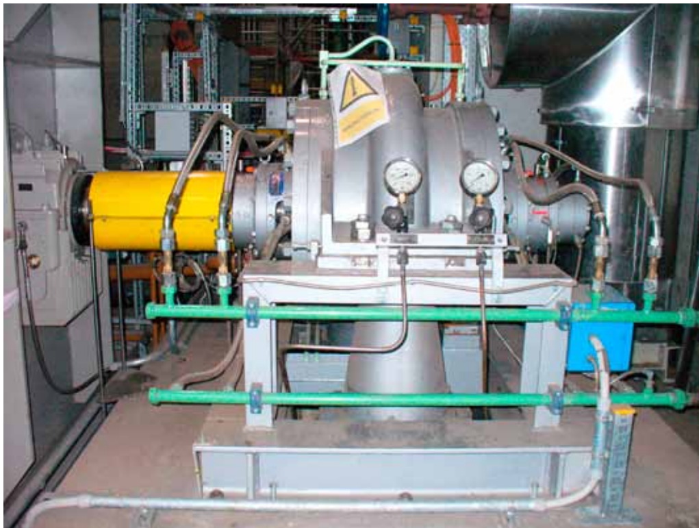
Booster pump 300-QHD, Coal-Fired Power Plant Ledvice (CZ)
